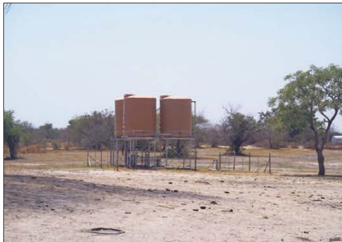
One of the many boreholes and water tanks located throughout the Eastern Caprivi that provide safe water
