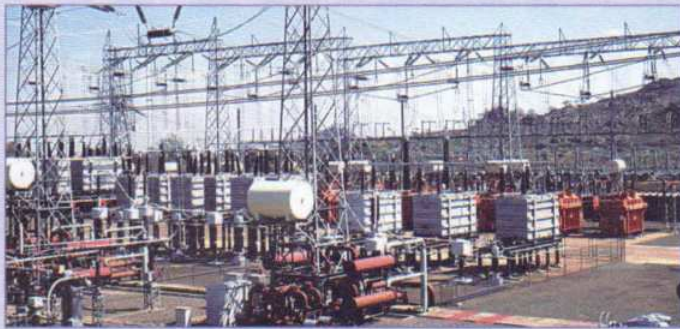
New transmission projects such as Zizabona are expected to ease congestion in existing central corridors in the region.
