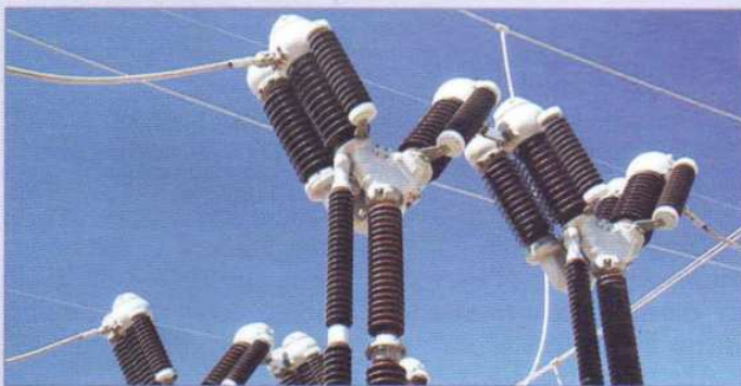
Regular inspection of interconnectors remains vital for preventing power transmission disturbances.
